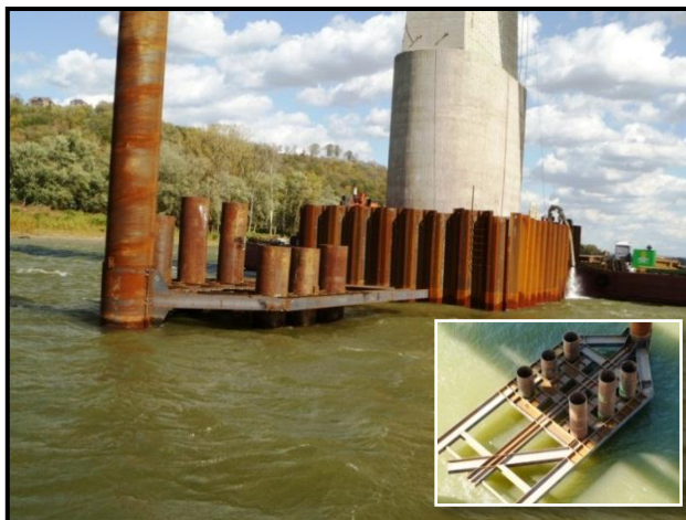
Temporary towers are being built just west of the existing piers. (Inset shows aerial view of towers.)
